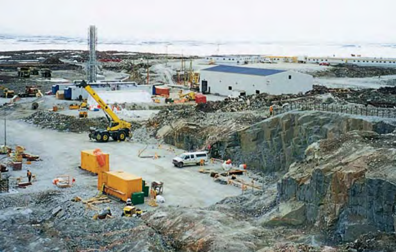
Figure 3. At the future Diavik diamond mine, a kimberlite processing plant is being constructed. The tower in the left center of the photo will be the exhaust stack for the processing plant, and the low, white buildings in the distance are temporary living quarters for 700 people. The four kimberlite pipes that will be mined are located under the shallow waters of the ice-covered Lac de Gras in the far distance. Photo taken on May 28, 2001, by K. A. Mychaluk.
