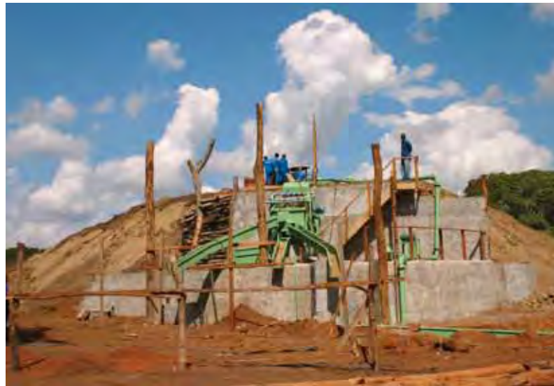
Figure 14. This washing plant, constructed by Mozambique Gems, will be able to process 150–200 tonnes of material per day when it is completed. Photo by J. C. Zwaan.
