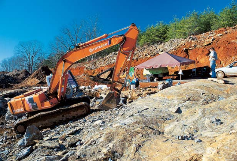
Figure 29. The weathered overburden in the back-ground has been removed to expose the gneiss hosting emerald-bearing fissures at this North Carolina emerald mine. Ground penetrating radar was then used to locate mineralized fissures. Photo by Robert Weldon.
